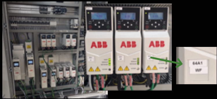
ON THE INVERTER DEDICATED TO THAT AXIS
